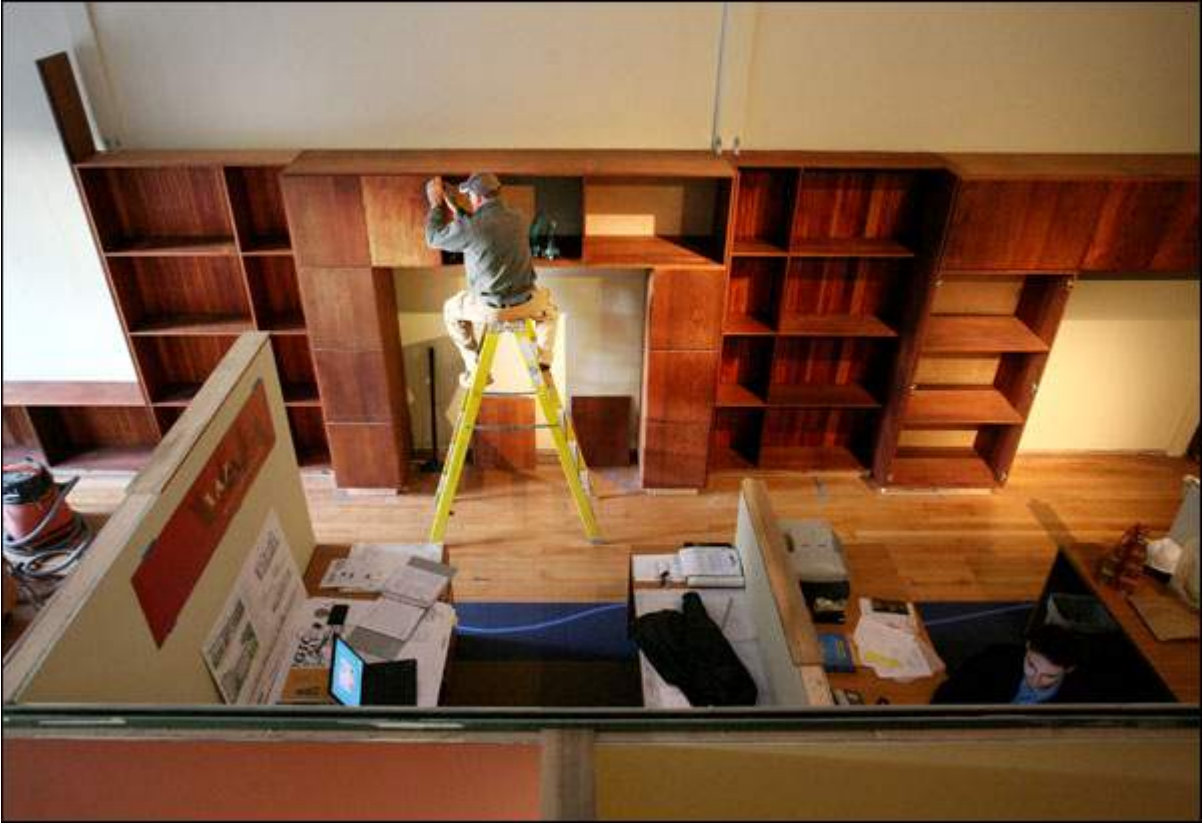
Randy Rissman installs cabinets recycled from redwood shelving salvaged from Petaluma's old silk mill at the new office of Wattenbarger Associates. Terry Hankins
